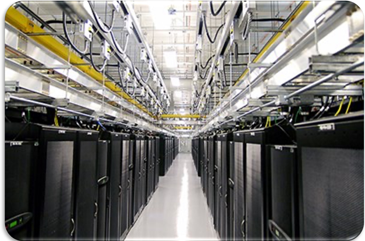
MGHPCC: Massachusetts Green High Performance Computing Center
